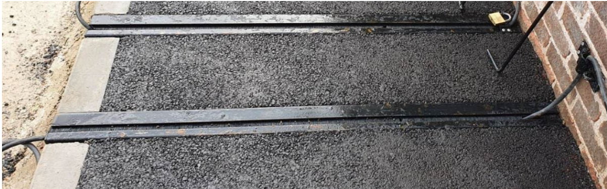
Picture 2 –A gulley channel (Gul-e project) for an EV charging cable provided by Oxford City Council
